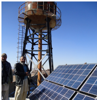
Figure 1.10: Solar water pump
