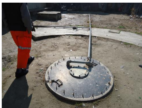
Picture .3 Koti Sangi Community Toilet Linked Biogas Plant (Courtesy of BORDA Afghanistan)
